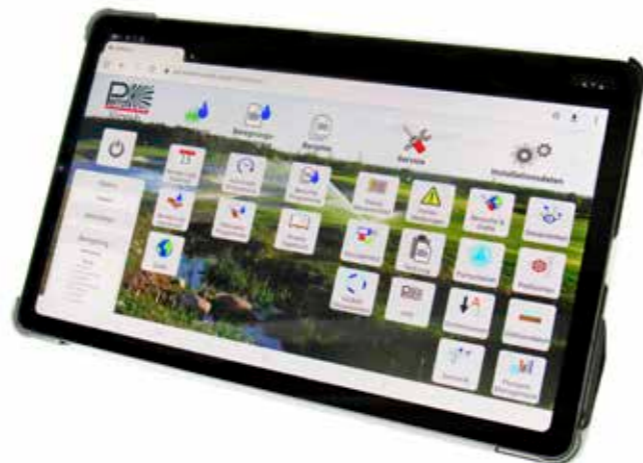
The control system can also be accessed via a tablet or smartphone.
