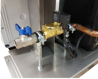
Quick fill 3/4" solenoid valve from incoming supply
