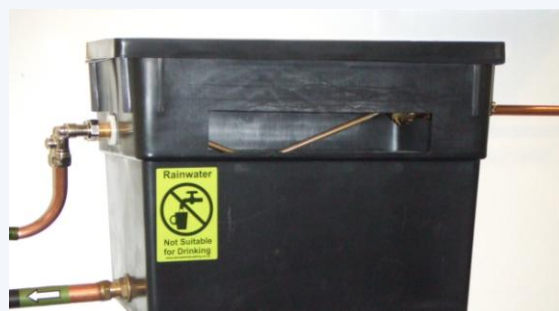
Figure 3: examples of labels for storage cisterns and point of use appliances e.g. washing machines, WCs, outside taps etc.
